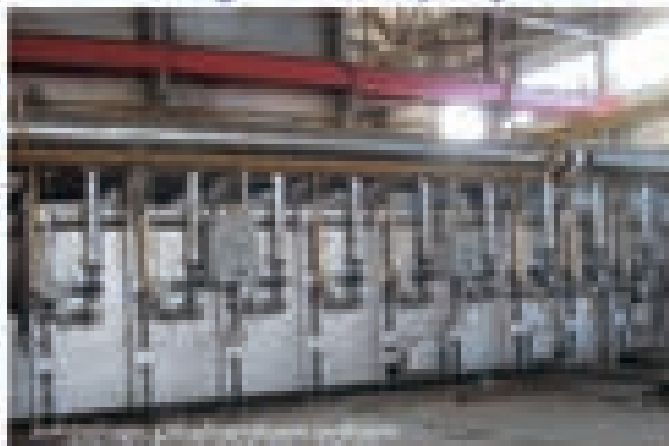
Inlet Reheating Furnace
